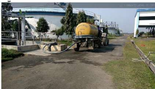
Inlet Pit and Digester
