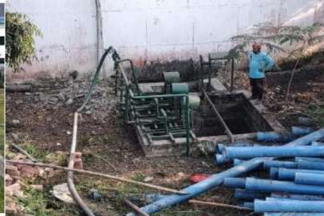
Digester Outlet Sump
