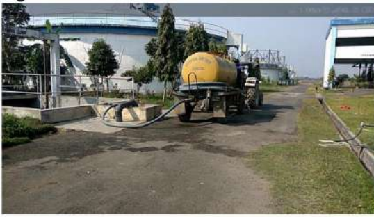
Inlet Pit and Digester
